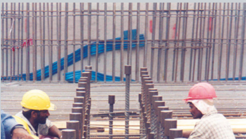
Bartec/Fortec couplers in columns
