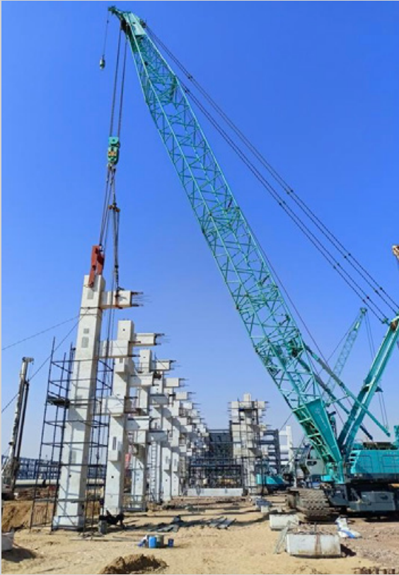
Groutec S Coupler in pipe racks
