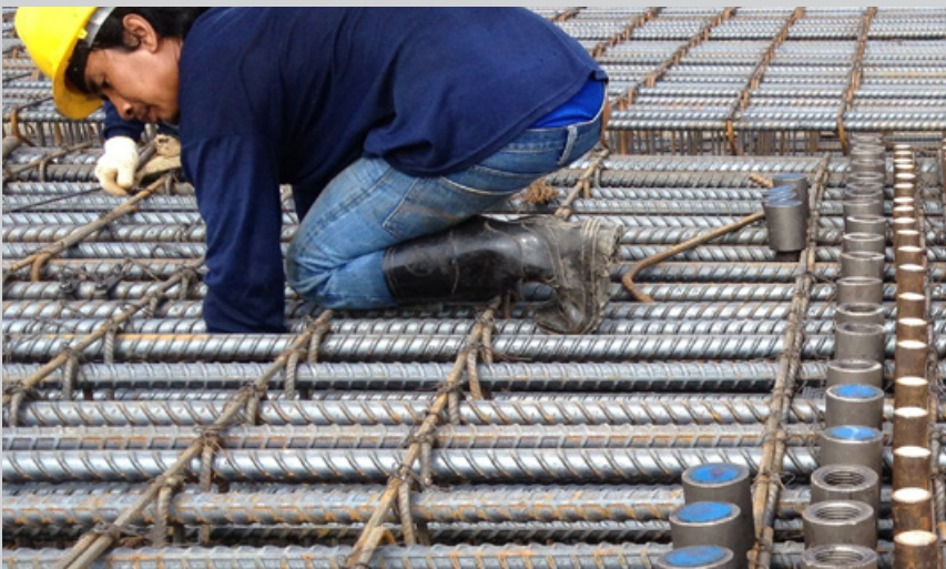
Bartec/Fortec couplers in columns.
